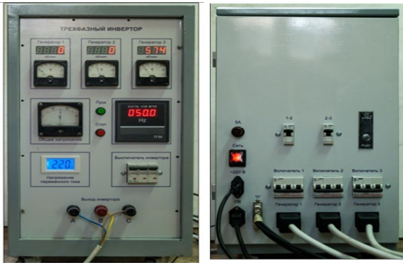
d) Front and rear panels of the three-phase inverter with measuring instruments
