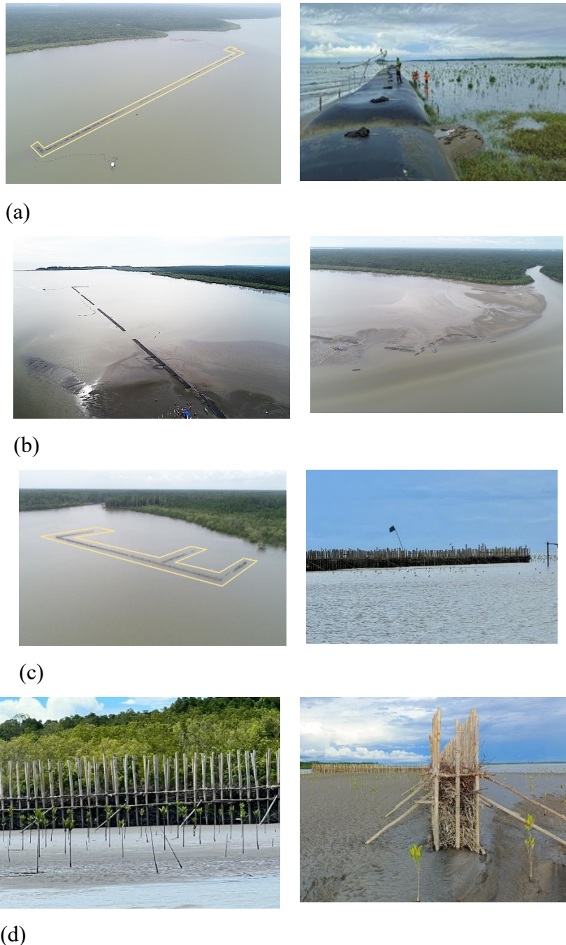
Figure 4: Estuary structures built in Ajkwa Estuary: (a) Geotube construction; (b) sedimentation occurred in the area of Geotube; (c) E-groin construction; (d) sedimentation occurred in the area of E-groin
