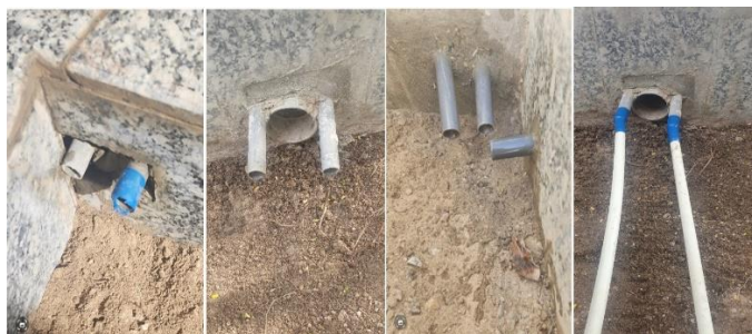
Figure 2: The AC drainage piping outlets
