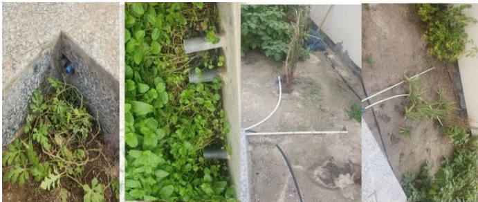
Figure 7: The outlets of the AC drainage piping extend out to the garden.
