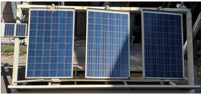
a) Solar Panels (Photovoltaic Modules)
