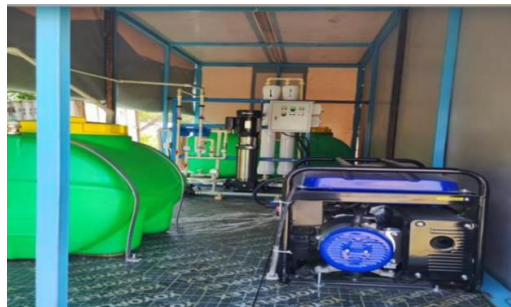
Figure 1: Interior view of the mobile desalination system
